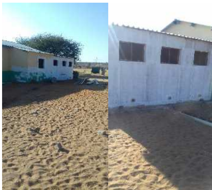
Progress so far, the girl’s toilets on the left and the boys on the right.
