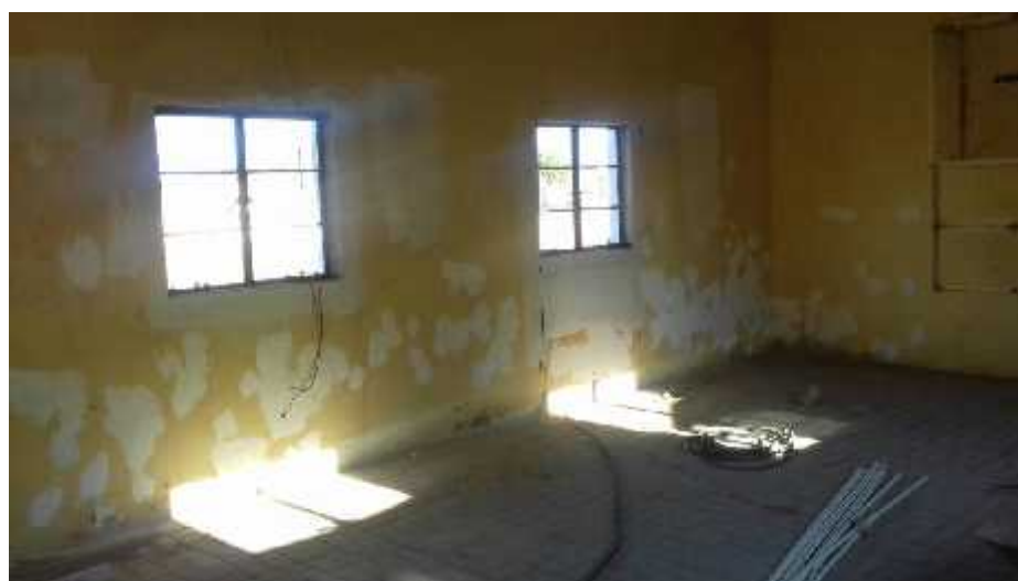
The installation of new windows as part of the conversion of a storeroom into a dormitory.
