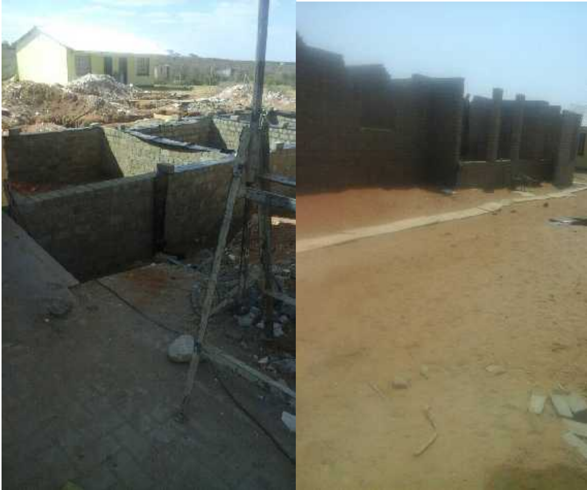
Construction work taking place at the clinic. (apologies for the quality of the picture on the right).
