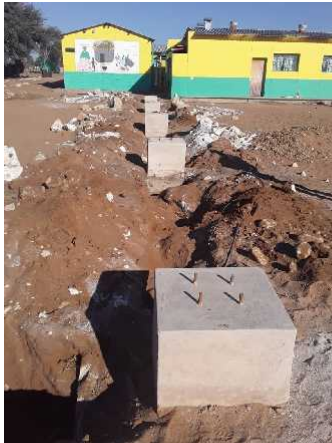
Some of the foundation blocks waiting for the erection of the steel uprights.
