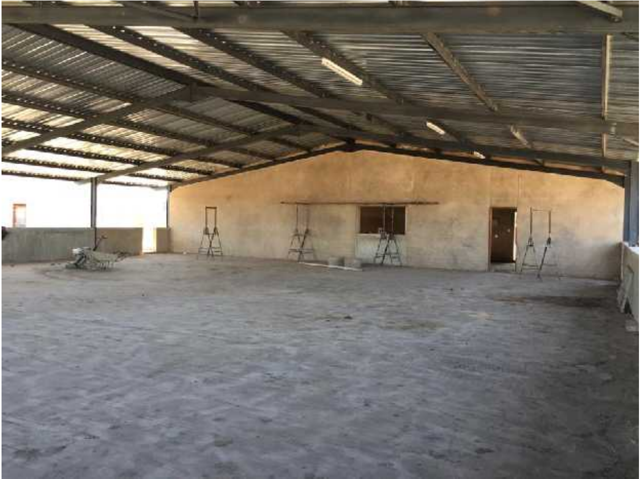
Photo showing progress in June 2016. Dining area awaiting paving and the kitchen was well on the way to completion.
