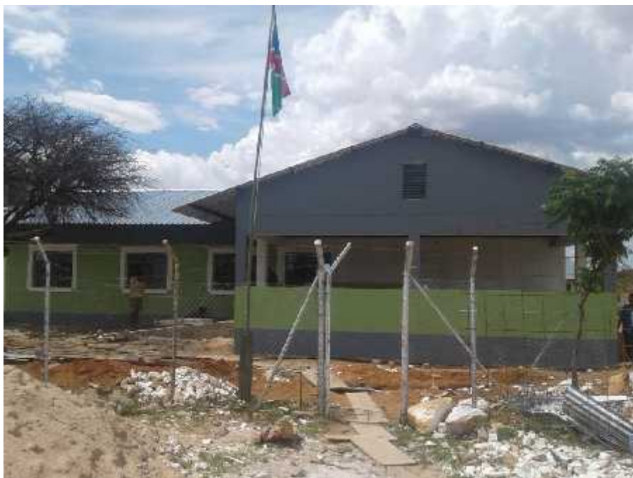
This photo show progress as at January 2018 and shows the Reception area
