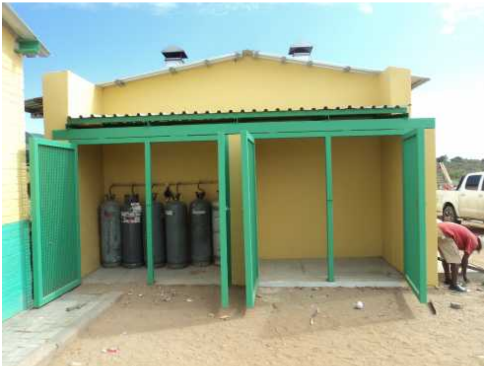
Gas ranges installed with the aluminium pots, while the lower picture shows the outside secure area for the gas cylinders.
