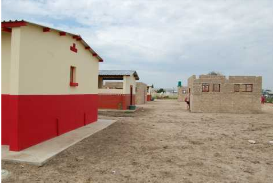
The three partially finished buildings of the NGSIP project, currently scheduled to complete in October 2014.
