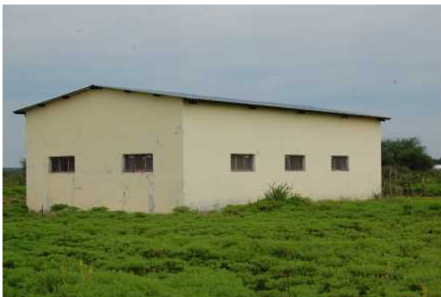
The shop/warehouse which is a possible candidate to convert to a kitchen and dining hall.
