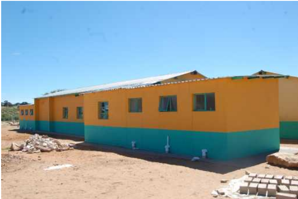
In the far left of the picture are the boy’s toilets, while the middle building is the new dormitory and to the right are the girl’s toilets.
