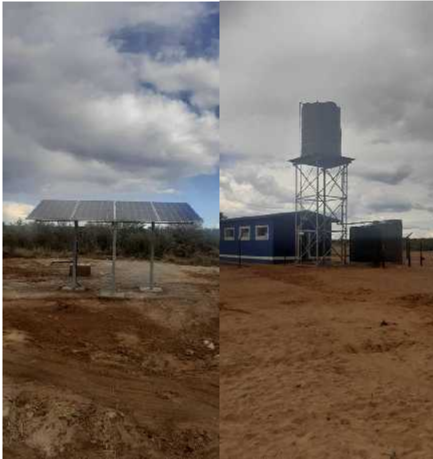
Left: The solar panels in place: Right: A new 10,000 litre tank on its stand beside the hostel.
