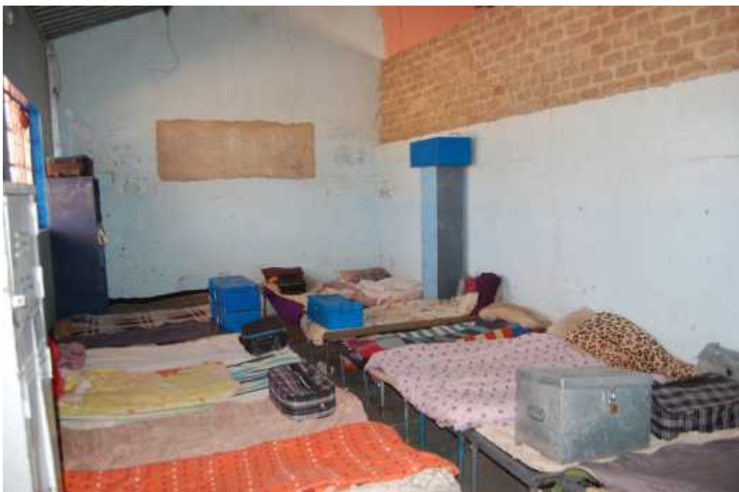
The boy's dormitory at Hippo Primary School in need of refurbishment
