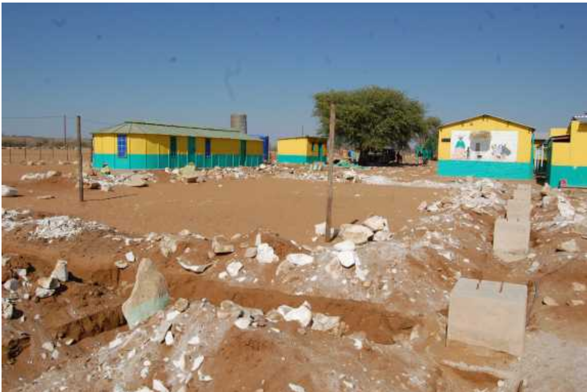
The foundations of the multi-purpose hall in October 2019 prior to work recommencing.
