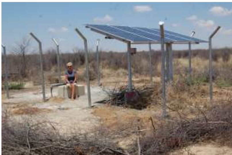
At last the construction of the fence has started with Linda having a Diana moment
