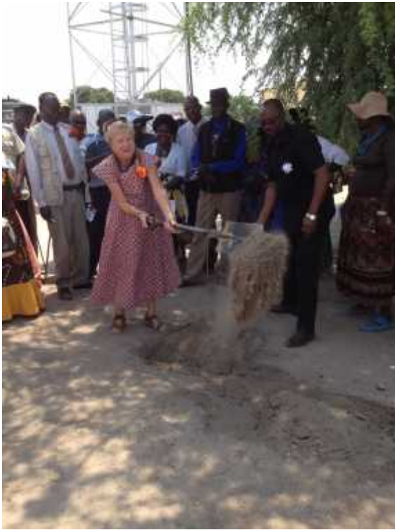
Linda and the Regional Governor, Mr Festus Ueitele carry out the ground breaking ceremony for the kitchen and covered dining area.
